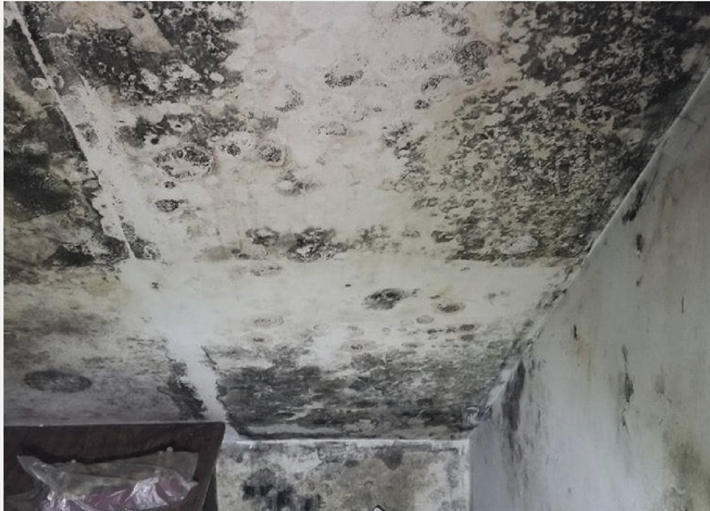
"wall tiles riddled with cracks and greenish buds of mould" (1)
